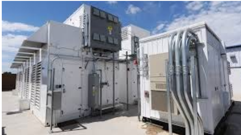
Figure 2b – Example of One Large Multi-Rack Enclosure
